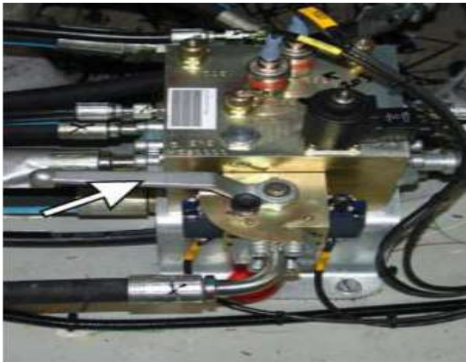
Figure 16-3: Shut-off valve on distribution block.
