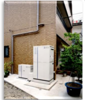
Tokyo Gas / Ebara
